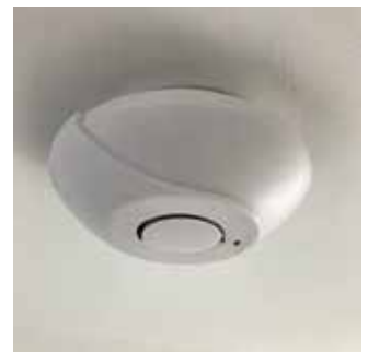
Mains smoke alarm
