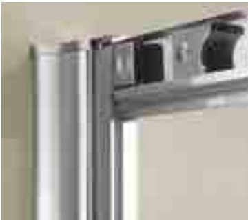
Minimal fixings inside
