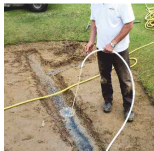
Testing of Enviroflow (1.00 pm)
