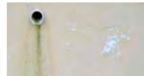
PAINTED, DAMP SUBSTRATE
