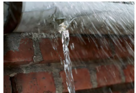
Leaking roofs or condensation from pipework
