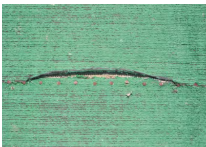
Unsuitable entrance matting
