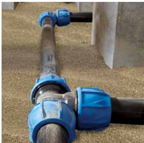
Water Distribution Lines
